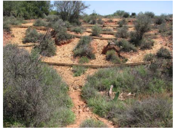
4. On steeper sites, the fences are installed netting in series down the slope. Note the areas of mulch between the fences.
