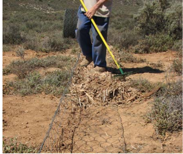
2. With the fence complete, a thick layer of mulch is applied over the full length of the fence.
