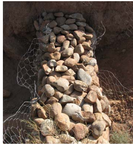
2. The trench is lined with wire netting and the gabion constructed with stones.
