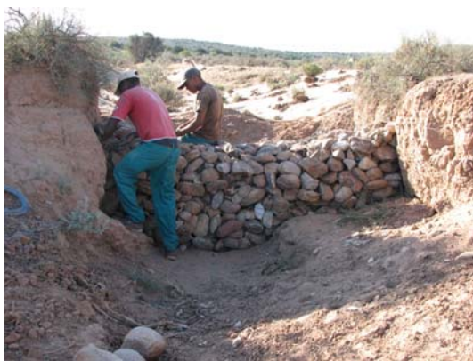
3. When at the correct height, the wire netting is closed tightly over the gabion.
